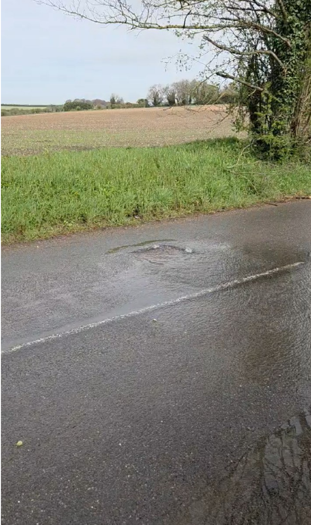
Figure 2: Evidence of sewer surcharging on Aldworth Road, adjacent to the Pumping Station, 4 th April 2026
