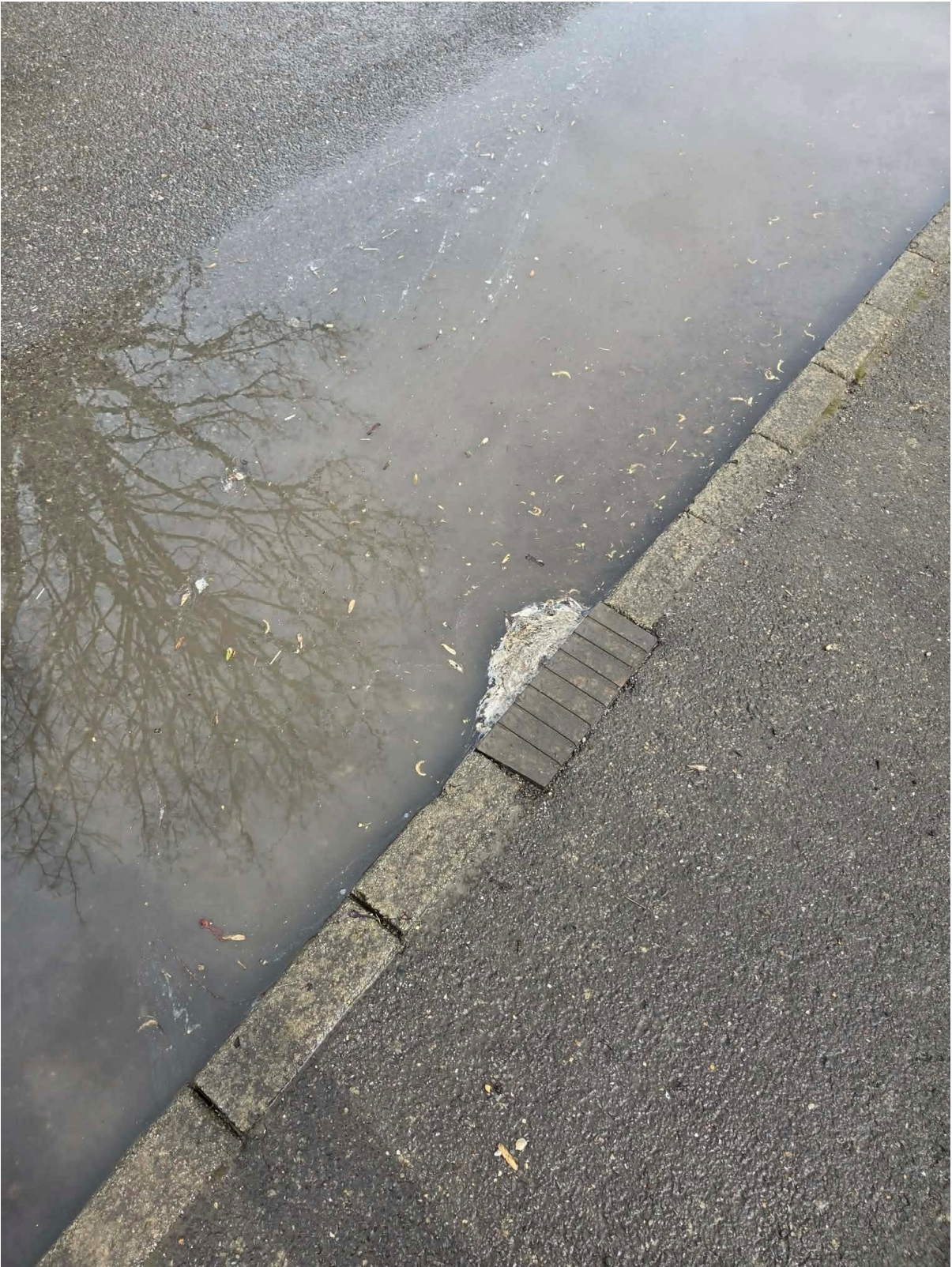
Figure 3: Evidence of surcharge residue on Aldworth Road adjacent to the pumping station, 4 th April 2026.
