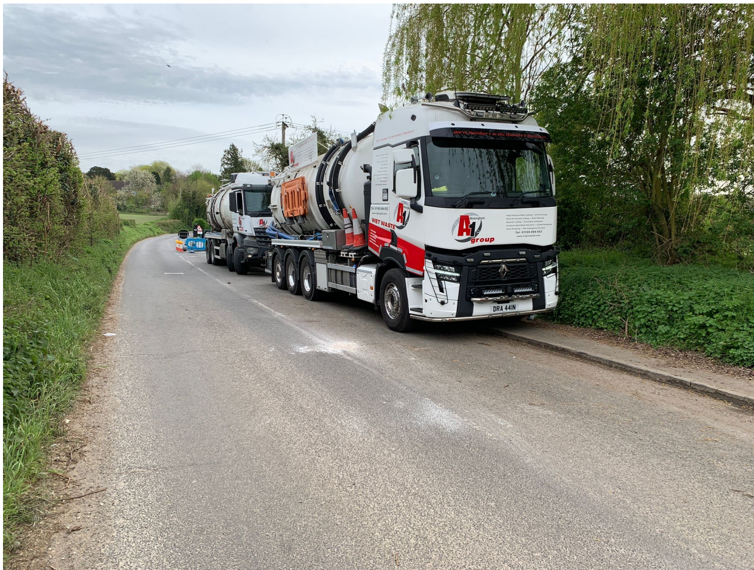
Figure 4: Two tankers stationed at Aldworth Road pumping station during ongoing network management, 9 th April 2026.
