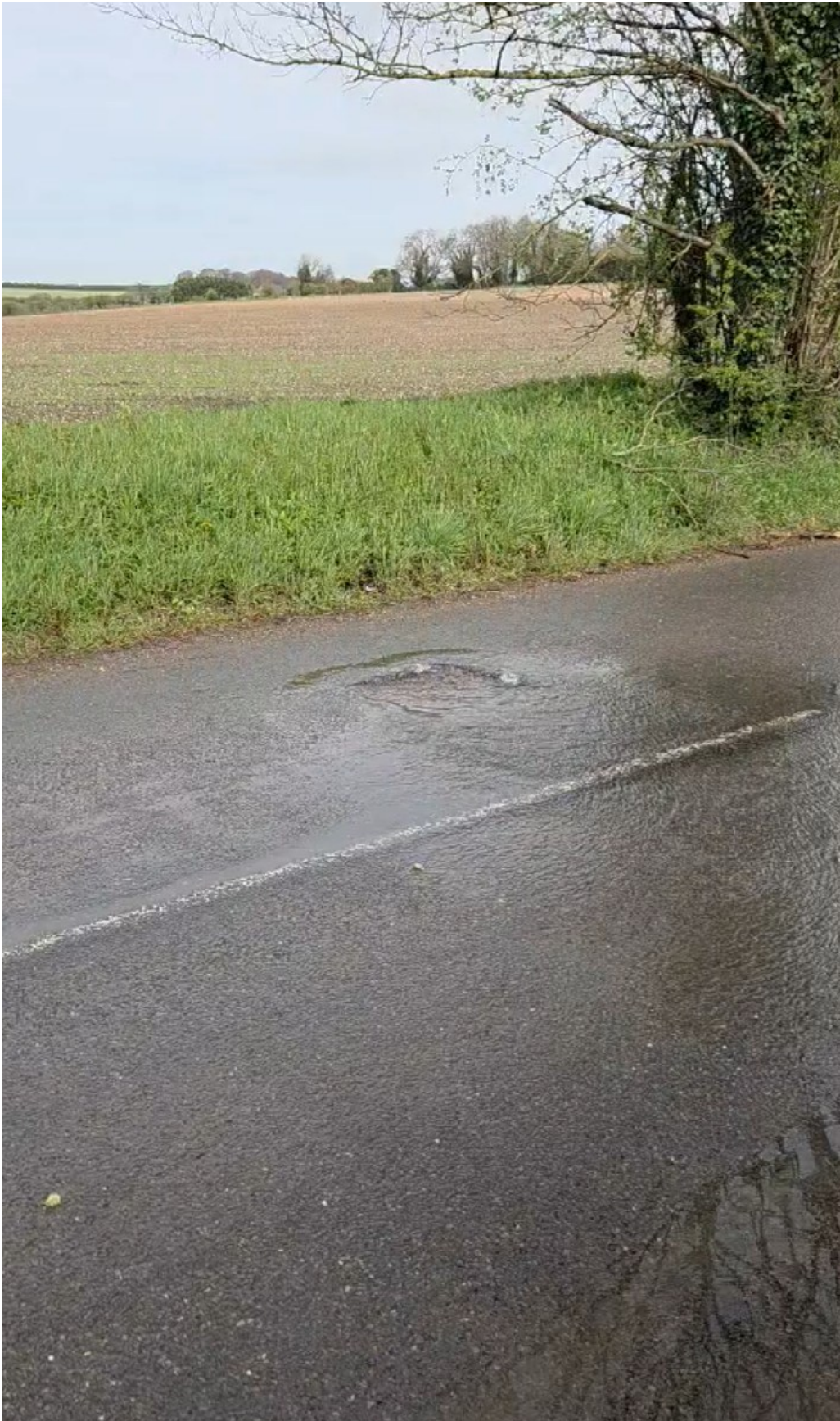
Figure 2: Evidence of sewer surcharging on Aldworth Road, adjacent to the Pumping Station, 4 th April 2026
